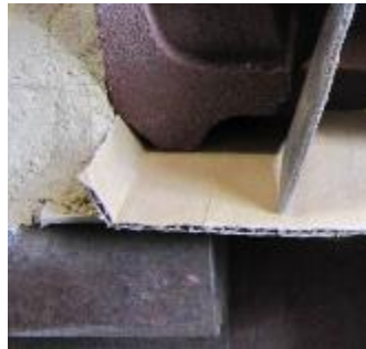
at worn rails
